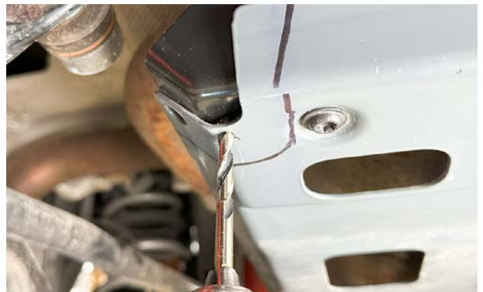
4. Use a 1/8" drill bit to drill a hole through the skid plate only.
