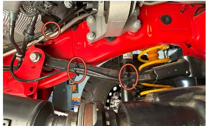
10. The front axle will require approx. 70" of tubing. Route the tubing as shown from the differential to the master cylinder located in the engine compartment. Secure the tubing at regular intervals using the provided zip ties. NOTE: Avoid routing the tubing alongside hot areas and avoid the steering shaft.
